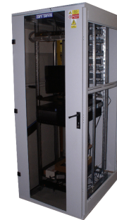
Rack with server, modems and UPS
